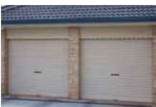
Examples of not approved garage doors
